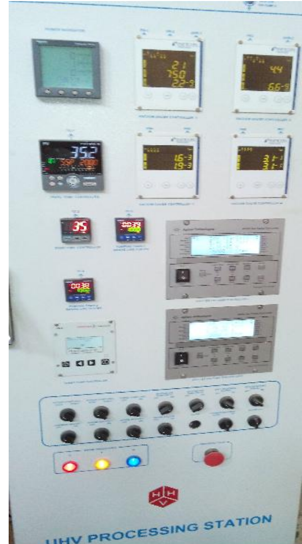
Vacuum station control unit
