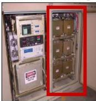
High Voltage Power Conditioning
